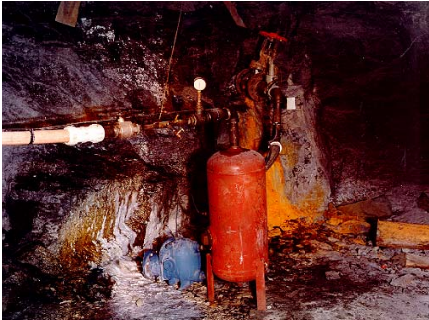
Figure 6. Post drilling water separation and safety and monitoring system implemented by REI Drilling, Inc. at boreholes at the Soldier Canyon Mine.
