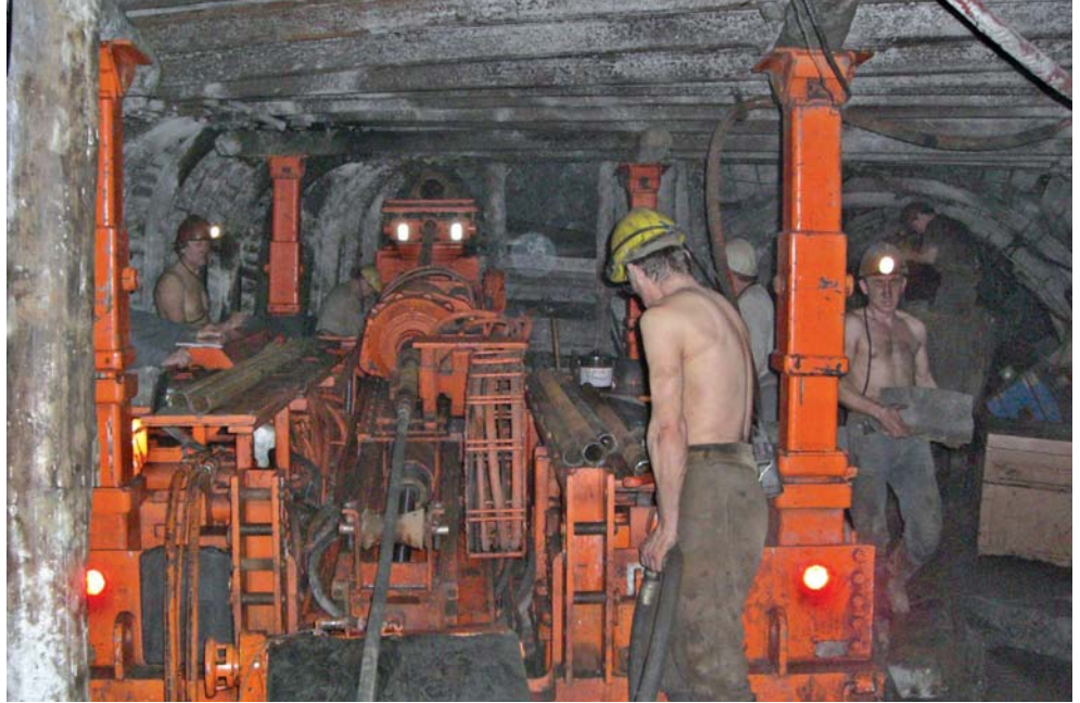
Figure 2: Directional drilling of horizontal gob boreholes underground at the Belozyorskaya Mine in Ukraine.
